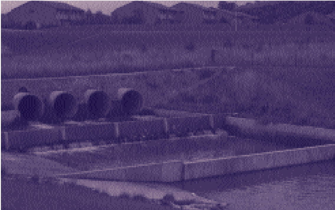
A gross pollutant trap in Kambah, ACT, collects coarse debris before it can make its way into urban ponds. Photo: Ian Lawrence
