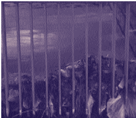
Gross pollutant trash rack.
