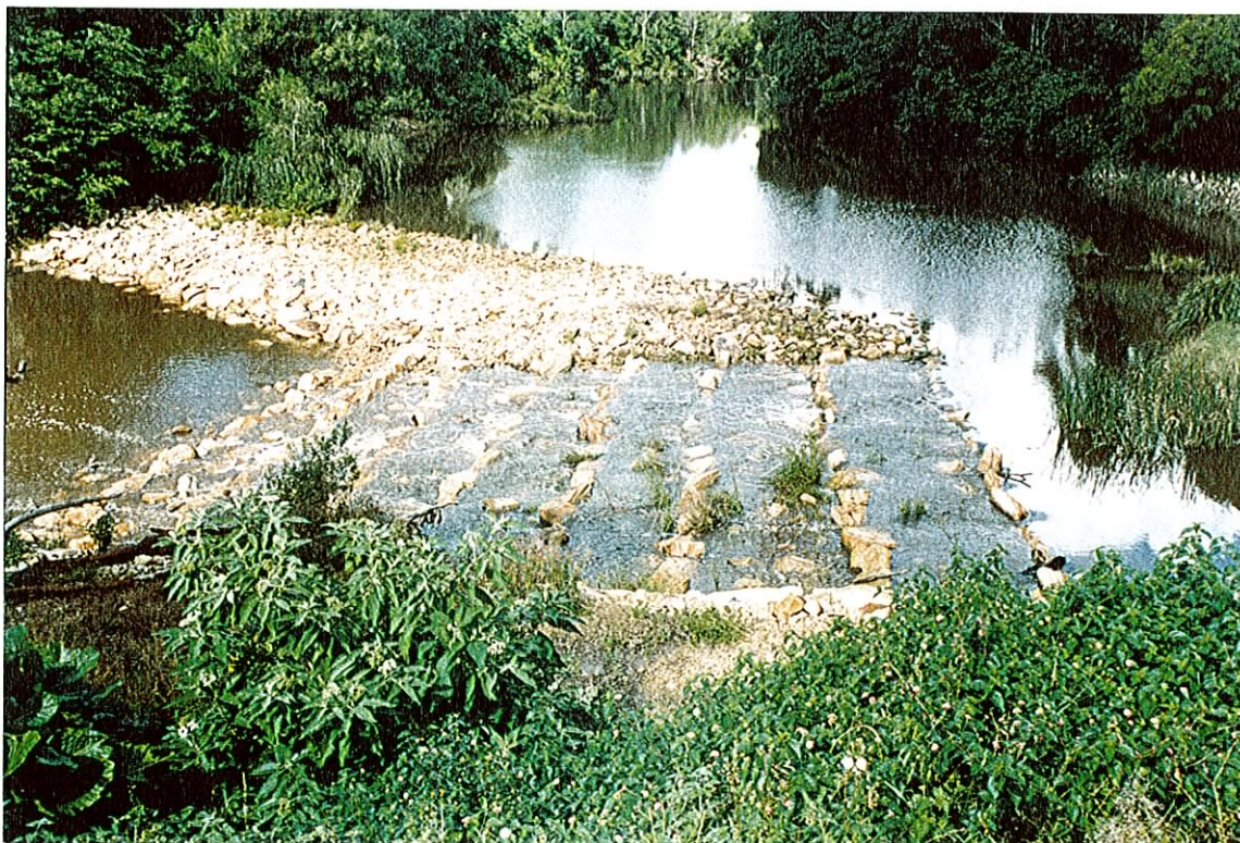
Photograph 6. In September 1993 extra rock was placed below the Lower Wyong Weir and a rock-ramp fishway formed. (Note the lower weir crest in the foreground)
