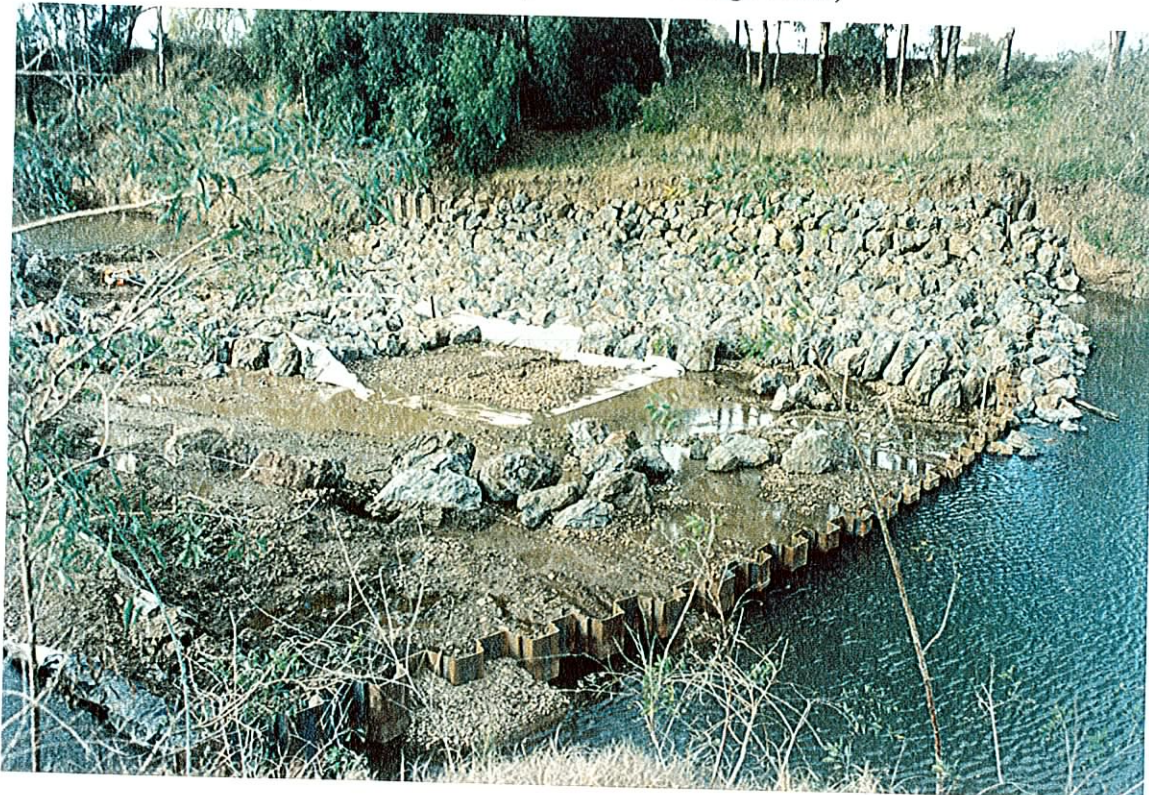
Photograph 7. The construction of a erosion control weir on the Bell River in June 1993. (Note the sheet-pile wall and the placement of large rocks)
