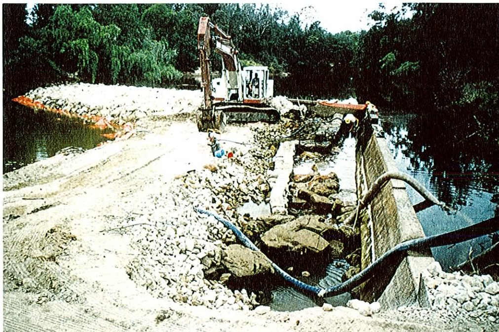
Photograph 5. The placement of rocks below the Lower Wyong Weir, Wyong River to prevent water leakage through the existing concrete structure.
