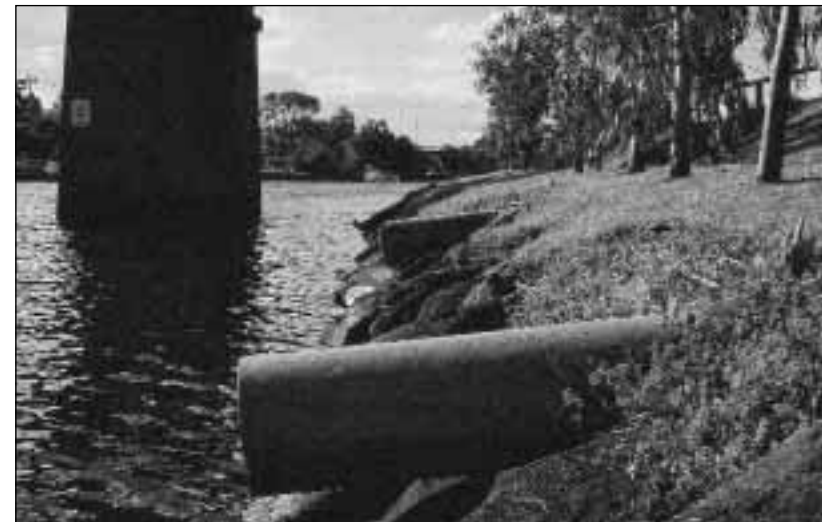
The urban stormwater drainage system includes underground pipes and open channels
