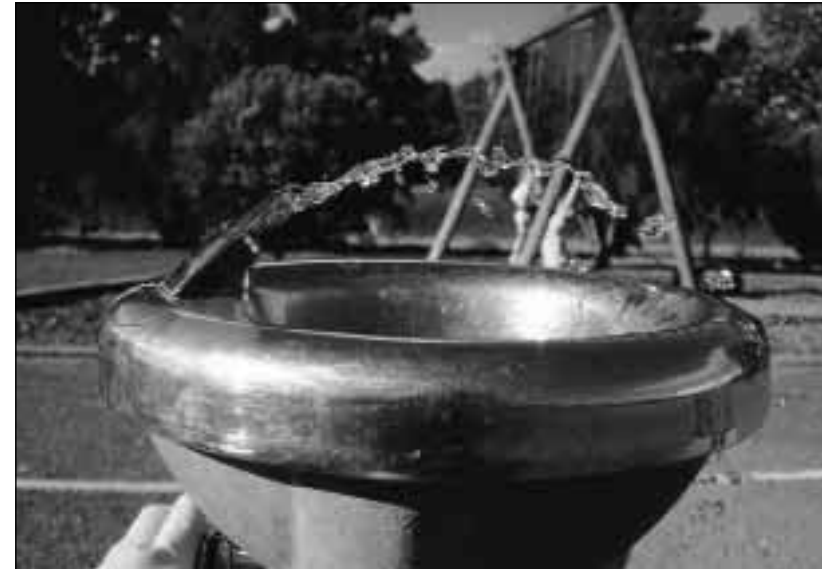
A large amount of infrastructure, from trunk mains to playground water fountains have been constructed
