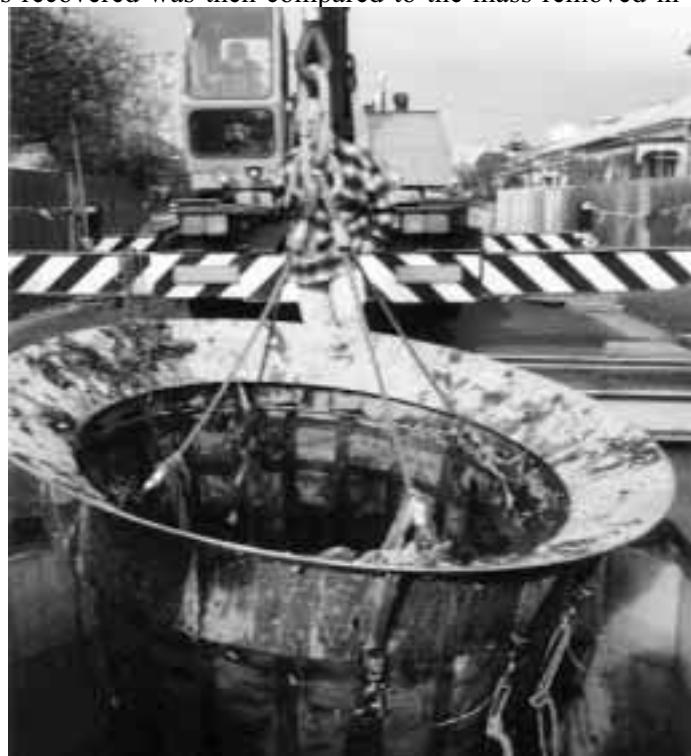
Photograph 7.2 Removing the sump-basket from the CDS unit
