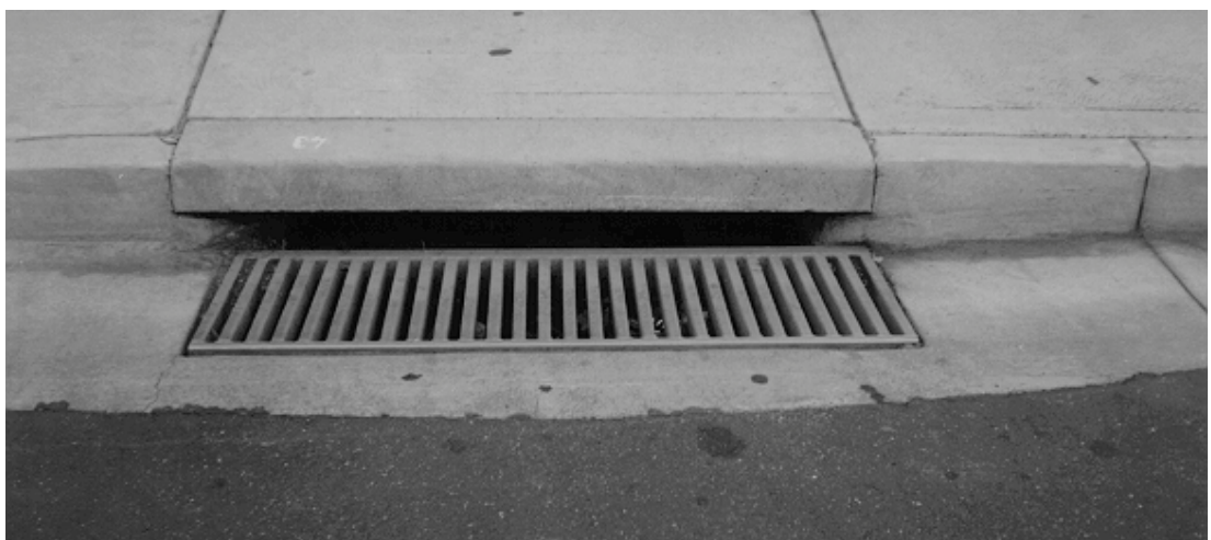
Photograph 8.3 A typical side entry pit with grate in the experimental catchment
