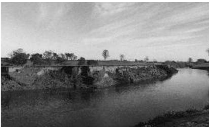
Figure 6.6: Topcliffe, the most downstream site on the River Swale (18 November 1995). The banks are approximately 4 m high, and flow is into the page.
