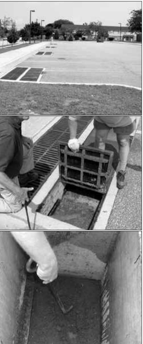
Figure 4.1 Below ground sand filters have been shown to be very effective in trapping grit and associated hydrocarbon – maintenance practice involves replacing of the top 50 to 75 mm of the sand every 3 to 4 years.
