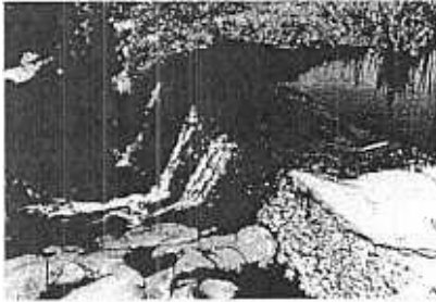
Figure 4.13: A fixed-crest weir in the Clyde River-Jervis Bay Basin (Cly 05).
