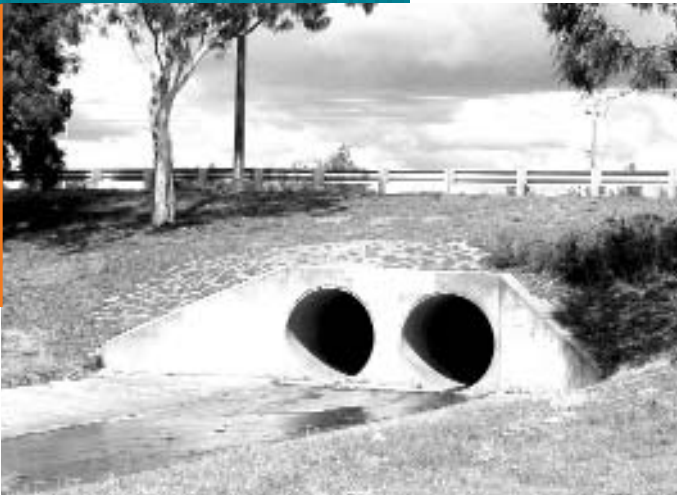
Stormwater pipes and concrete-lined drain leading directly to a stream, Belconnen, Canberra. Photo: B Rennie.
