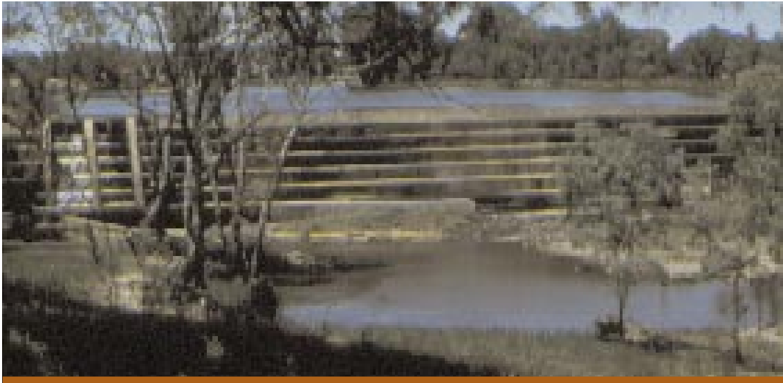
Campaspe Weir. The weir provides water for irrigation during the summer. Photo: Jane Gowns
