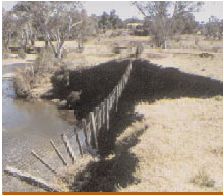
Bank erosion on the Gwydir River, Upper Darling system, near Bundarra. Recent work by the CRCFE has revealed that river regulation is a major contributing factor to bank erosion.
