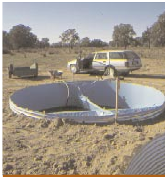
Constructing the artificial billabongs that were used in an experiment that investigated the effects of different inundation patterns on invertebrates and aquatic plants. Photo: Daryl Nielsen
