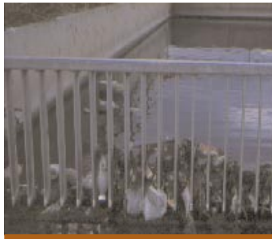
A gross pollutant trap captures an assortment of 'trash' from urban stormwater before it can enter ponds, wetlands and lakes. Photo: Karen Markwort
