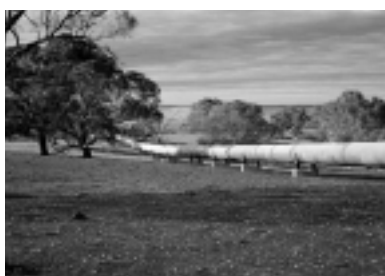
The Murray Bridge-Onkaparinga pipeline is one of three pipelines that take water from the lower Murray to supplement Adelaide's supplies. Photo: D Eastburn
