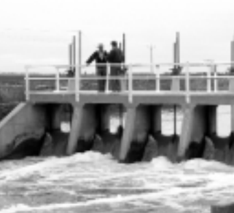
Supply channel flow and level control, Murrumbidgee Irrigation Area, NSW. Photo: B van Aken, CSIRO Land and Water
