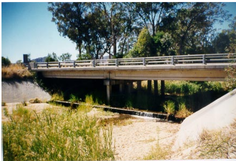
Fig. 4.5. Creightons Creek at the Hume Freeway Bridge. The concrete sill visible in the photo is a bed control structure that is protecting the bridge piers from being undermined.
