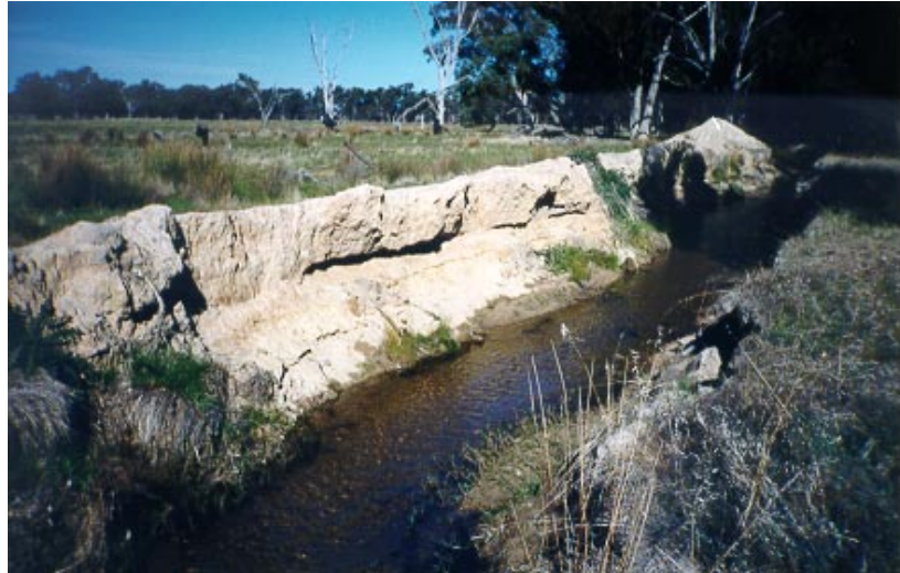
Fig. 5.5. Eroding stream-banks in the lower reaches of Creightons Creek
