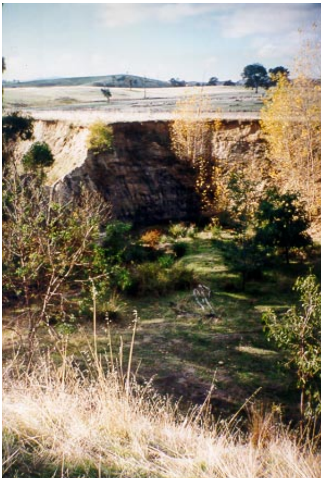
Fig. 4.10. Castle Creek upstream of the McLeans' property. Severe stream incision and widening has led to the formation of this chasm since the 1960s.
