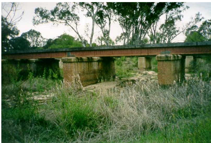
Fig. 4.13. Pranjip Creek at the railway line (Pranjip West Bridge). The stream bed in this vicinity has aggraded and degraded during the period since European settlement.
