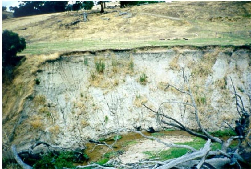
Fig. 5.6. Bank erosion on Creightons Creek due to undercutting
