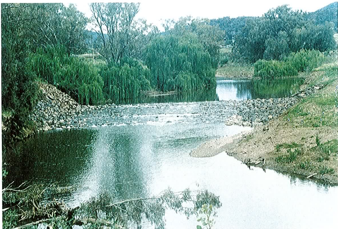
Photograph 8. After construction of the erosion control weir on the Bell River. (Note the rock-ramp fishway was formed in the centre of the structure)
