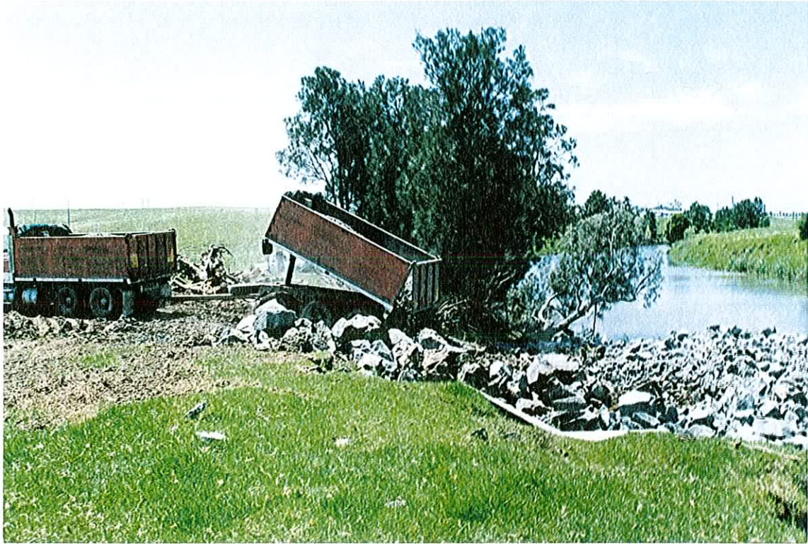
Photograph 1. Dumping of rock on site during construction of a rock-ramp fishway on McDonald's Weir, Macquarie Rivulet in January 1993.
