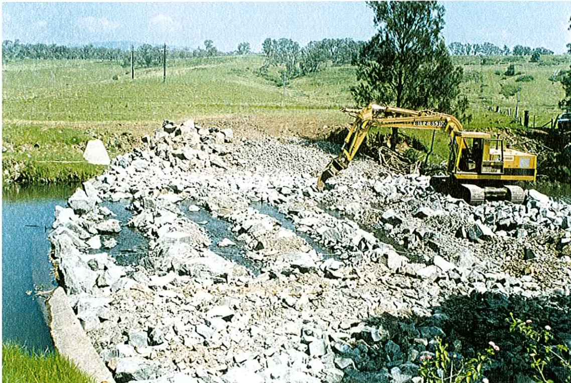
Photograph 2. Shaping transverse rock ridges during construction of a rock-ramp fishway on McDonald's Weir, Macquarie Rivulet.
