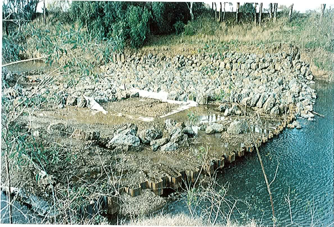
Photograph 7. The construction of an erosion control weir on the Bell River in June 1993. (Note the sheet-pile wall and the placement of large rocks)
